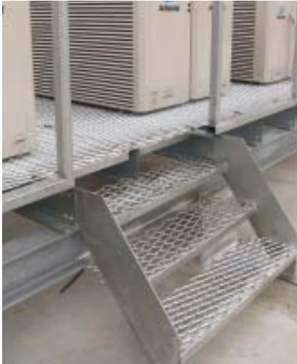
Air conditioning platforms
